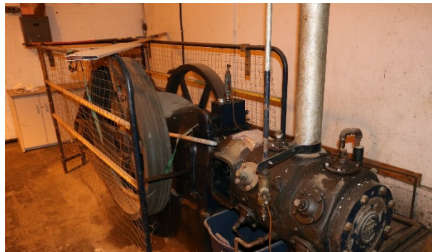
An incredibly powerful compressor used to supply air power for numerous air tools amongst other things
